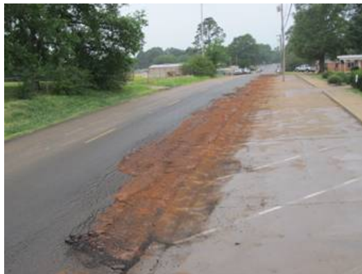
Damage from heavy trucks turning onto West Carolanne
